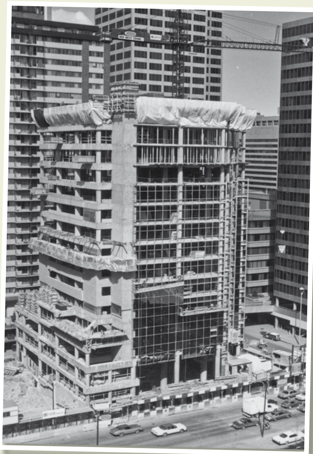
Construction of Chevron Plaza at 5 Ave. and 4 St. S.W. in Calgary in 1981.
