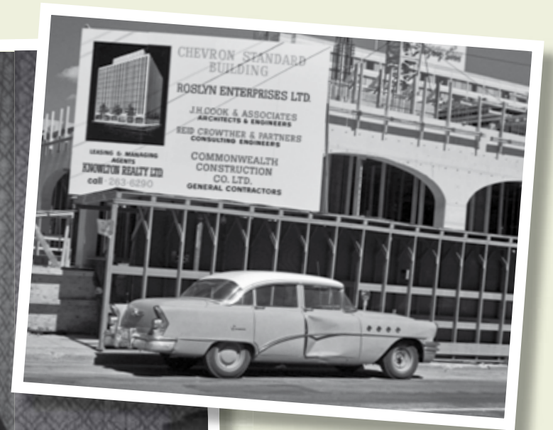
The Chevron Standard Building under construction at 5 Ave. and 3 St. S.W. in Calgary. The building was completed in 1967.
