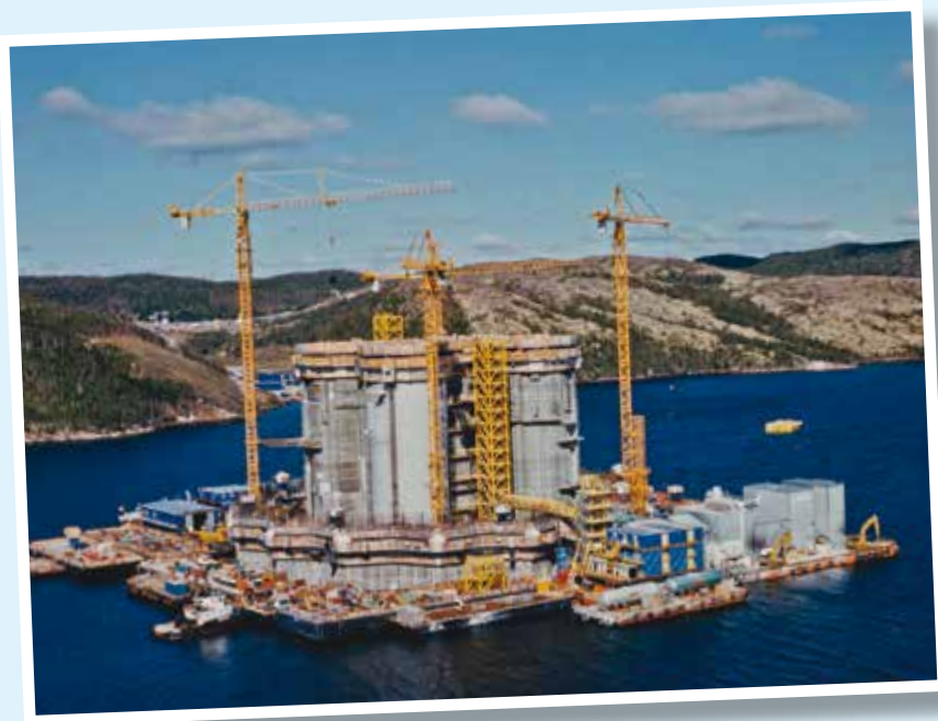
Construction crews work on the Hibernia gravity-based structure at Bull Arm, Newfoundland and Labrador, in 1995.
