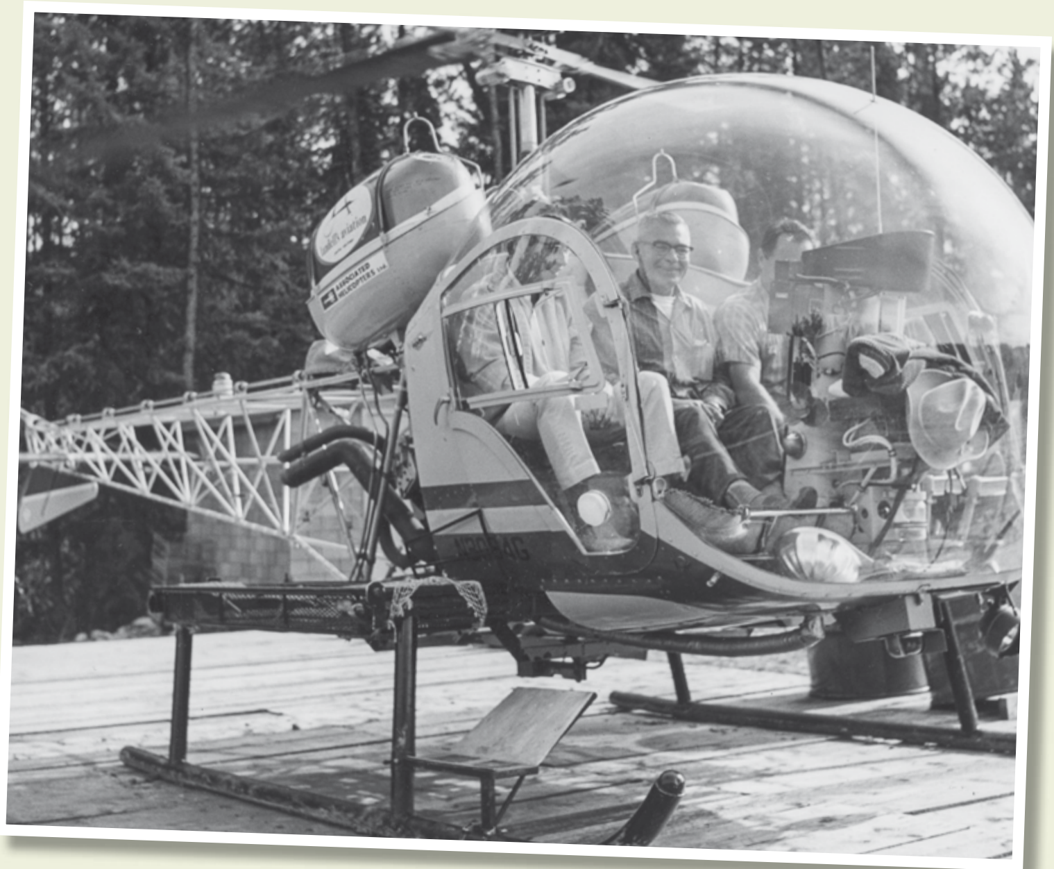
A helicopter supports construction of the Kaybob South Gas Plant in west-central Alberta.
